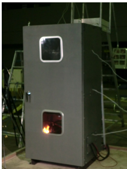
鉛蓄電池延焼状況①
